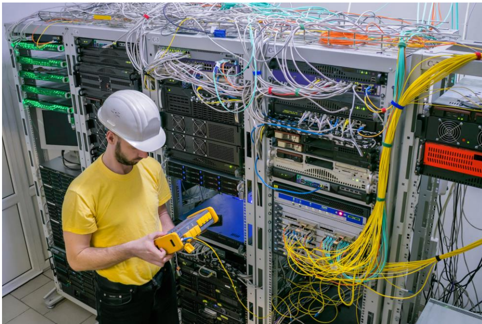
Fig 3.1.1.5 (h): Technician performing OTDR test
