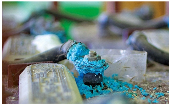
Fig. 2.5.14 Corrosion on the Battery Terminals
