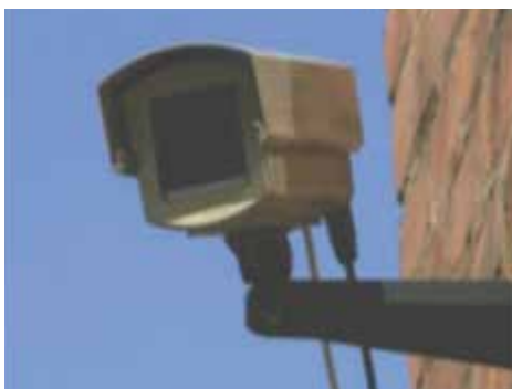
STEP 5: Placing CCTV Cameras at appropriate locations
